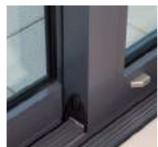
Threshold Where the situation allows, the threshold can be recessed into the floor level.
